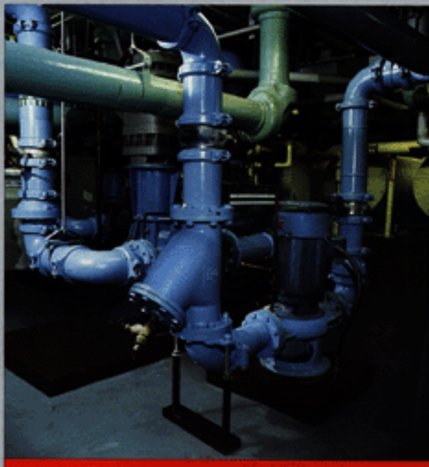
15 Floor Mounted Type VL In-Line Pumps supplying chilled and condensed water.—A major high-rise hotel at Baltimore's Inner Harbor
